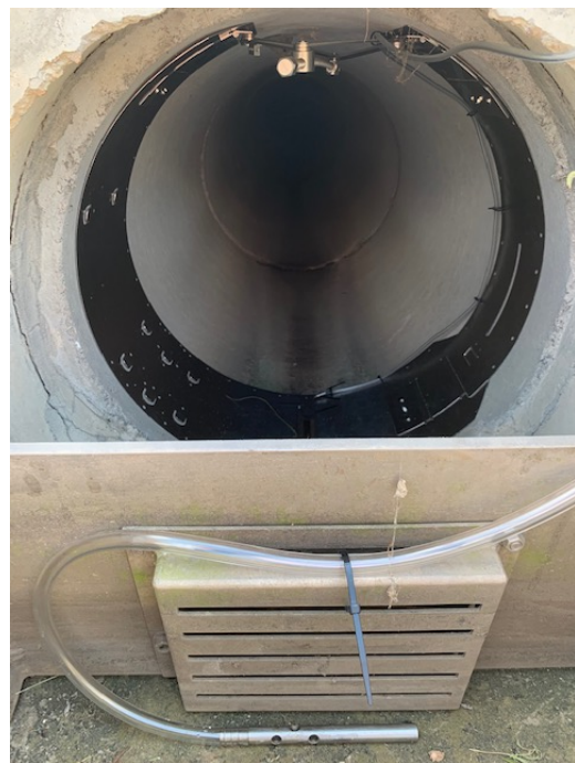
Figure 10. Set up at UTRP outflow pipe with control structure
