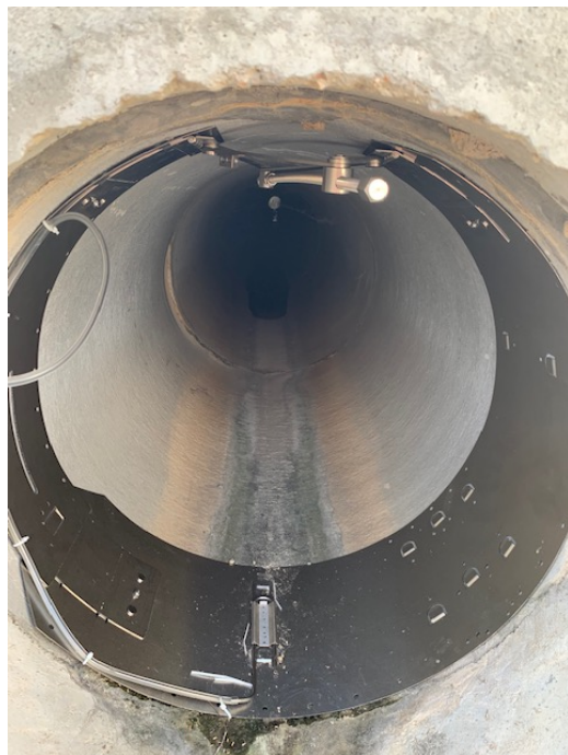
Figure 9. Set up at UTRP in the inflow pipe
