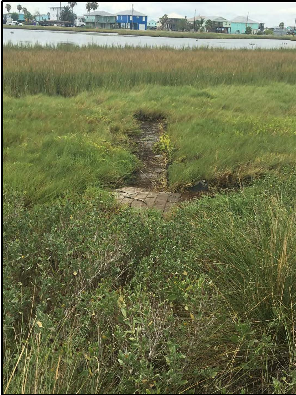
Example of what area of fringe marsh looked like with a section of roof over the vegetation
