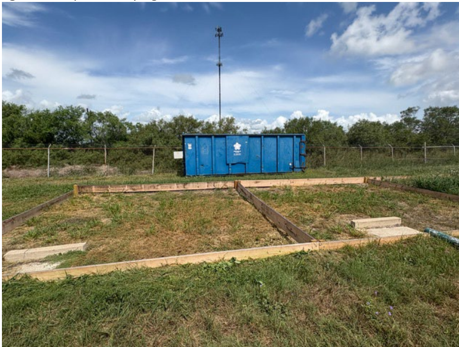
Figure 4: Replacement blowers at the Driscoll WWTP
