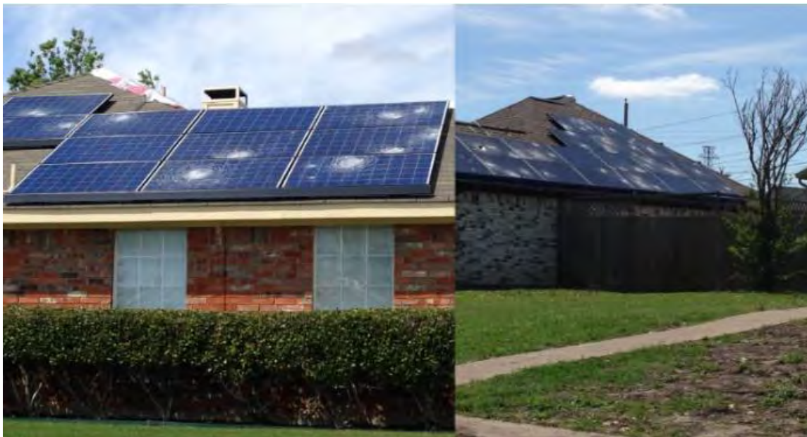
Figure 3-46: Hail damage to residential solar panels. 216
